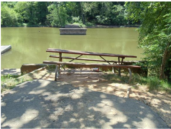
Dilapidated picnic bench
